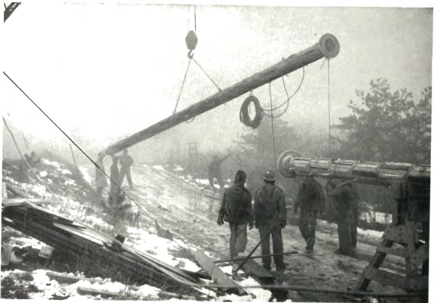
Unloading and assembling operations proceed despite cold and rainy weather. Here the top section of the antenna is being lowered into place so that the complete antenna can be assembled for a ground check at the WBRE-TV site.
