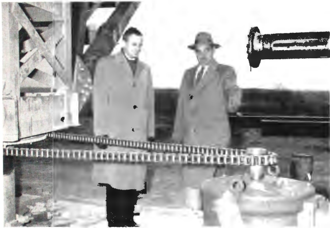
Messrs. Baltimore and Hopkins look over the drive mechanism for the 15-ton turntable. Remotely operated from the control and instrument shack shown below, the electric motor will drive the turntable from 1 to 5 rpm.
