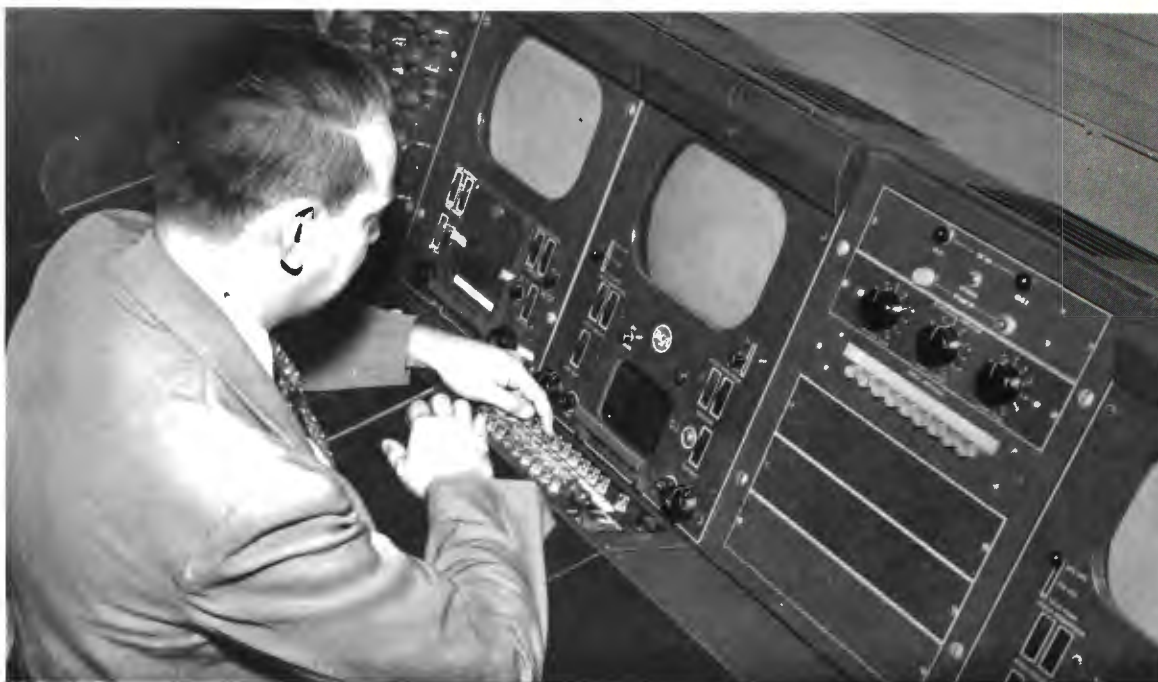
FIG. 29. View of the new TS-11A Video Switching Panel shown mounted in the sloping desk section of a typical Control Console. The TS-11A provides 9 inputs and 3 rows of push buttons for fades, lap dissolves and super-positions.
