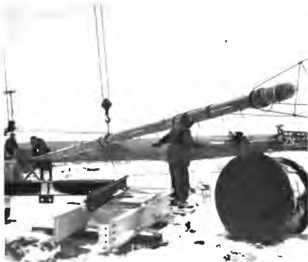
Top section is raised to be set inside the tower where it is joined to the bottom section.
