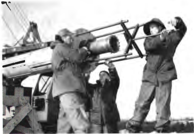
Using a specially designed harness puller, antenna workmen remove the harness for a very careful check before the two antenna sections are fitted together and raised to the 15-ton turntable for measurements.
