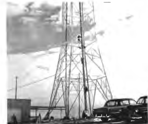
Completely assembled ultragain Pylon is suspended in the center of the TV tower.
