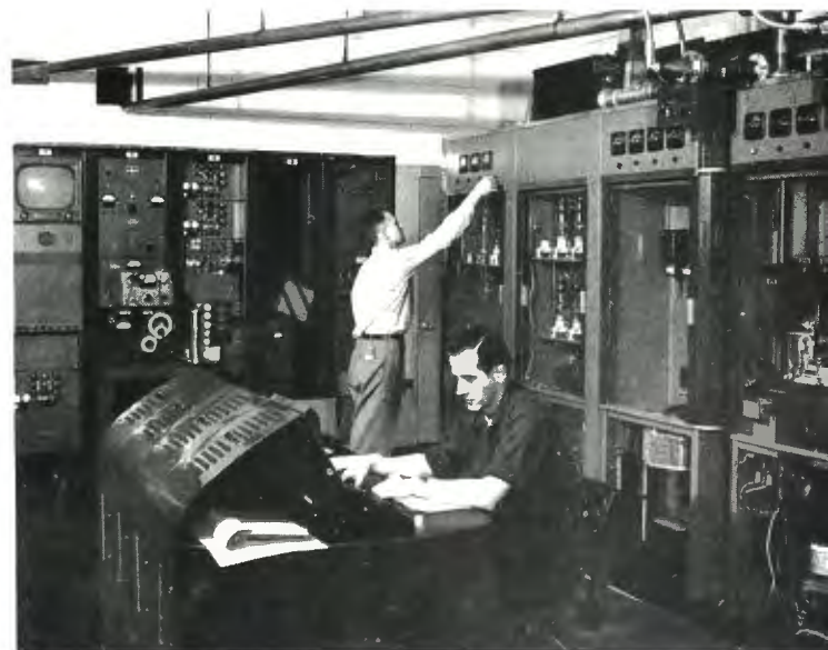
View of the WBRE-TV transmitter room. Four of the TTU-25A Amplifier cubicles are shown at the right. The station's original TTU-12A transmitter (not shown) is placed parallel to these cubicles about six feet to the front of the supervisory console. Transmitter equipment cabinet racks are pictured at the far end of the transmitter room.
